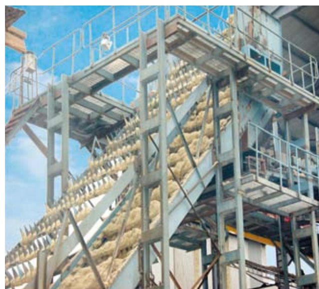
Bagasse conveying elevator
