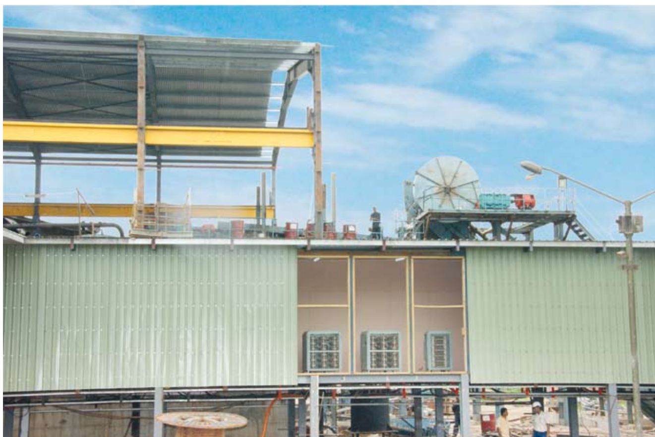
New control room for the new cane carrier at Rarawai Mill
