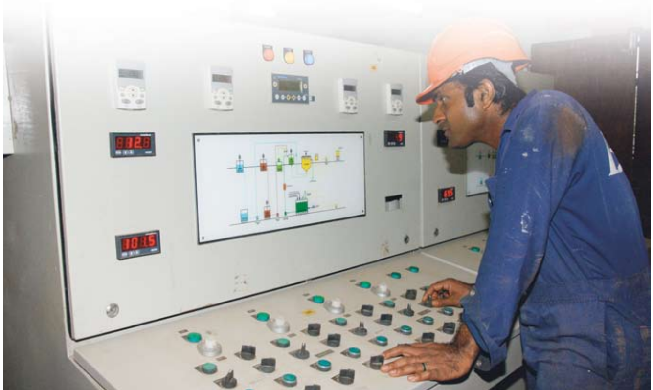
New control room for filtrate & syrup clarification system at Lautoka Mill
